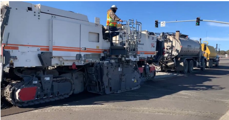
Front of CIR Train – Emulsion, Water & Grinder (11/9/2020)
