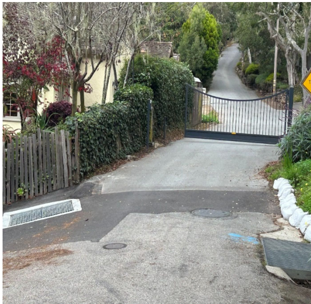
Completed storm drain catch basin at Second Avenue and Monte Verde Street.
