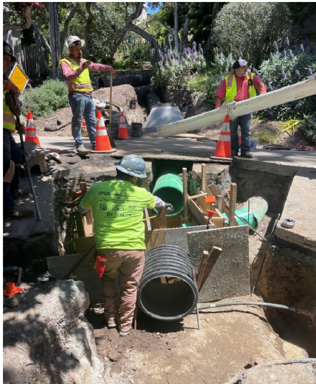
Construction of the catch basin at Second Avenue and Monte Verde Street.
