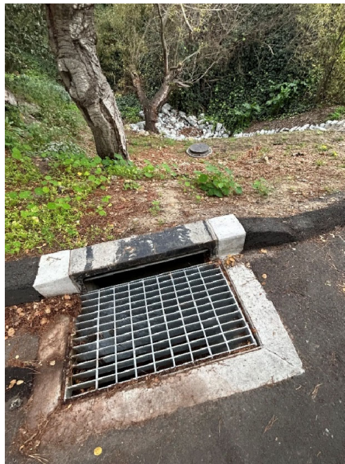
Completed drainage inlet at the south end of Santa Fe to the drainage channel outfall.
