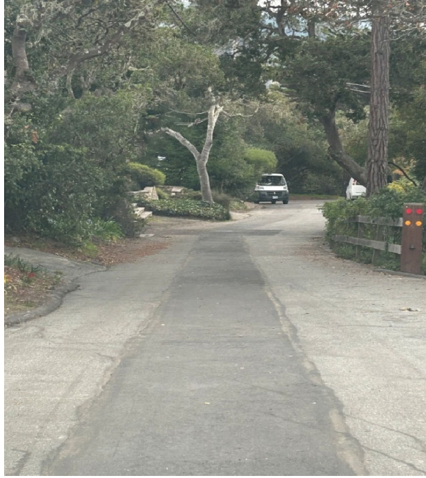
Completed SD pipeline along Santa Fe from 8 th Avenue to the MNTP Outfall.
