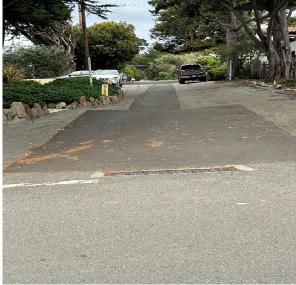
Completed Storm Drain Pipeline along 11 th Ave: Carmelo to San Antonio Streets
