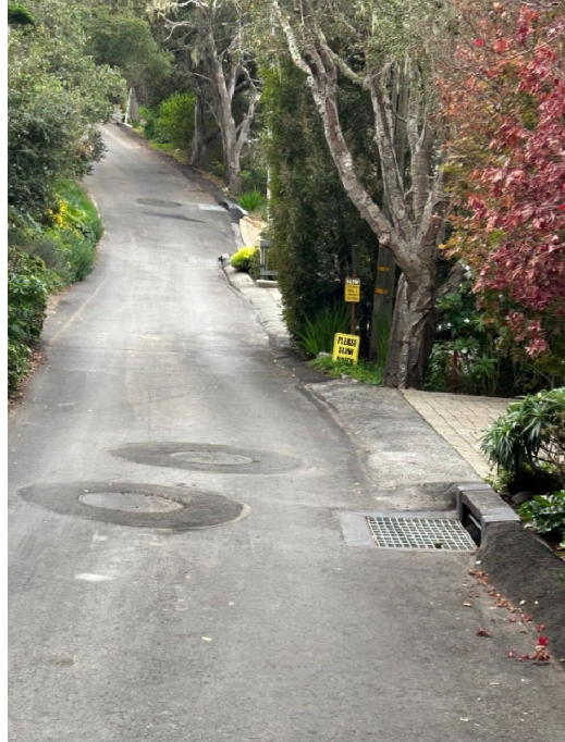
Completed storm drainage pipeline, manhole and catch basin along Lincoln Street (1st to 2nd Avenues).
