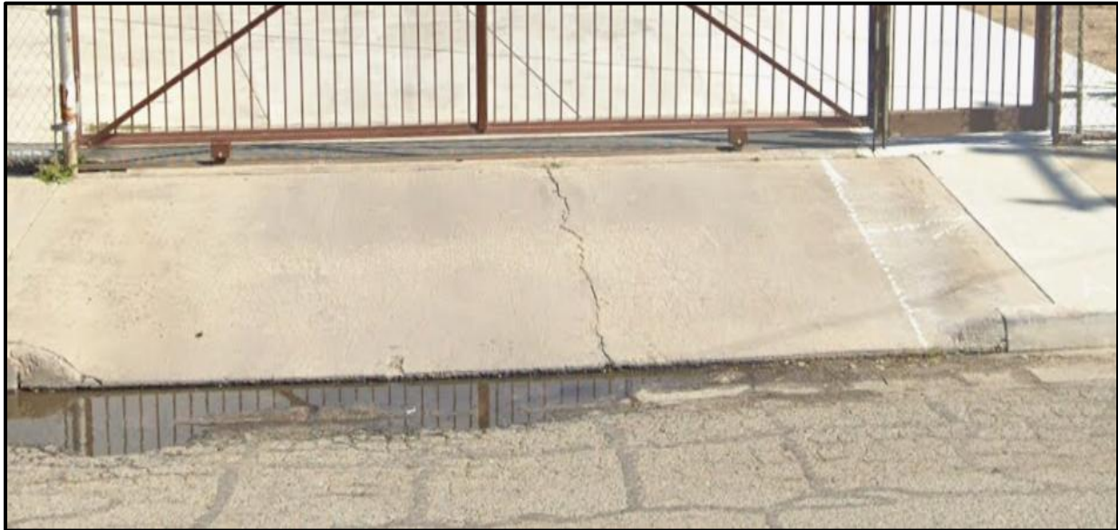
Figure 7 - State Street Sidewalk Repair Before Picture
