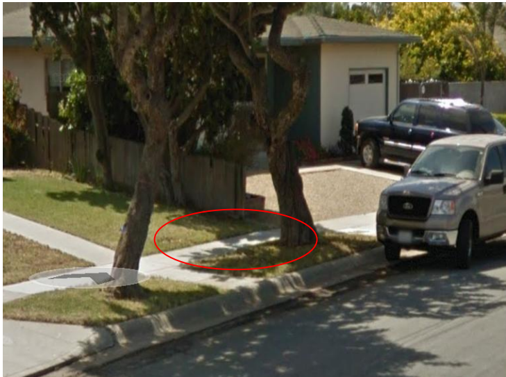
Figure 4 - Before: Tree Root Uplift at 522 Soledad St.
