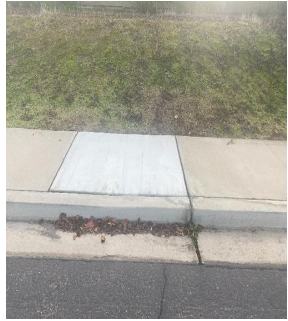
Figure 7 – After: Tree Root Uplift at Engstrom St
