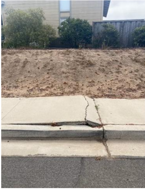
Figure 6 - Before: Tree Root Uplift at Engstrom St.
