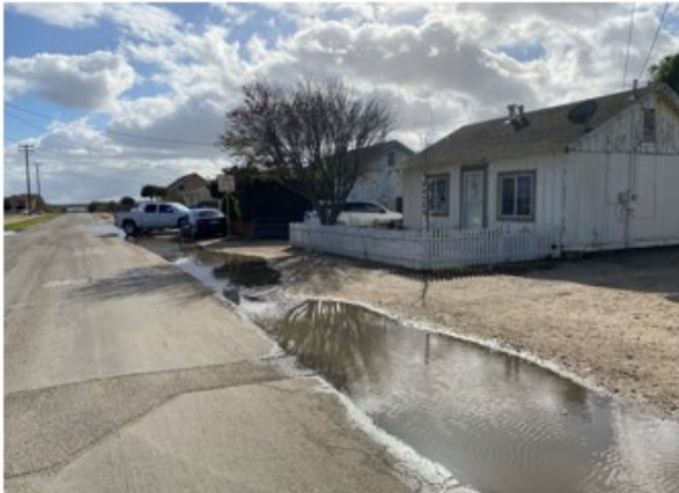
Before (Drainage issues, No sidewalk)
