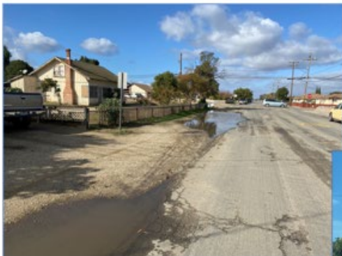
Before (Drainage issues, No sidewalk)
