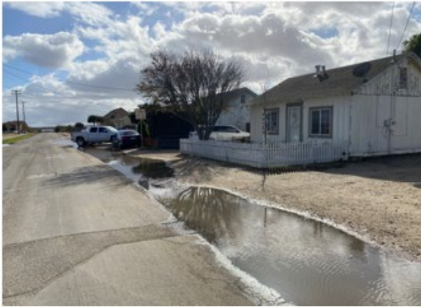
Before (Drainage issues, No sidewalk)
