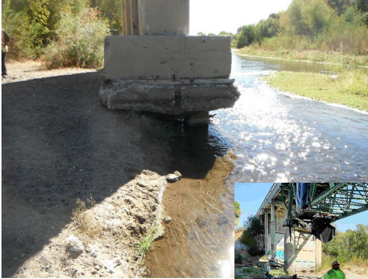
Scour of existing foundation
